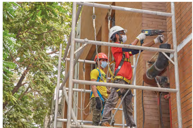
■ Maintenance work @ Dhaka Factory, BAT Bangladesh following all safety measures of EH&S
