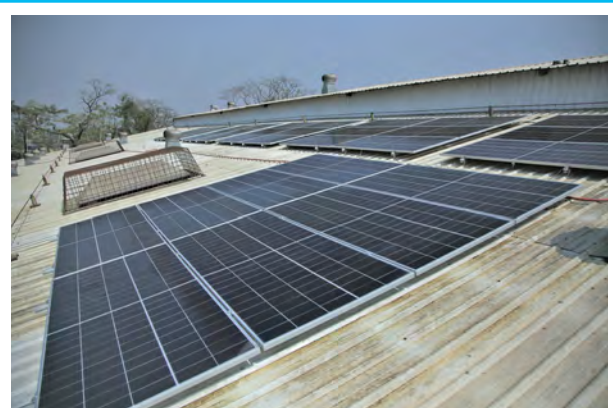
■ Solar Photovoltaic Power Plants for Enhancing Power Generation
