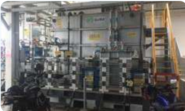
STP in Dhaka factory premises
