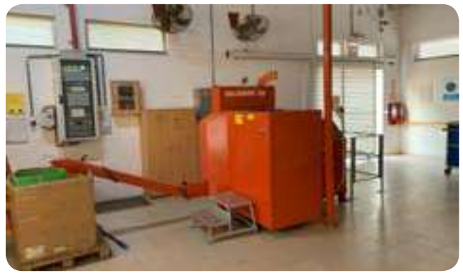
Briquette machine in briquette room
